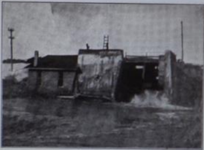
PELLSTON, MICH. The downstream wall (Bulkhead) of an open turbine penstock fell out into tail race in February, 1912. The bulkhead was badly designed and constructed. It had no reinforcing steel in it and the concrete was mixed of gravel and sand taken out of an old river bed. The plant was then in receiver's hands and has since been sold to the Cheboygan, Michigan, Light and Power Company and will be repaired this spring.
